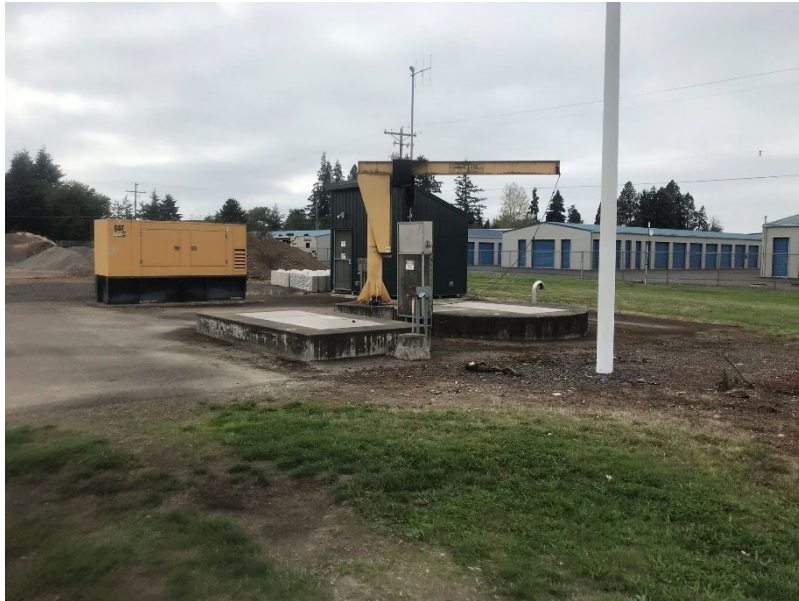
Figure 4-7 | Existing Influent Pump Station
