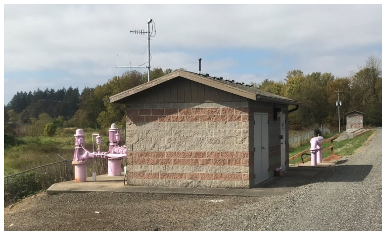
Figure 4-12 | Irrigation Pump Station
